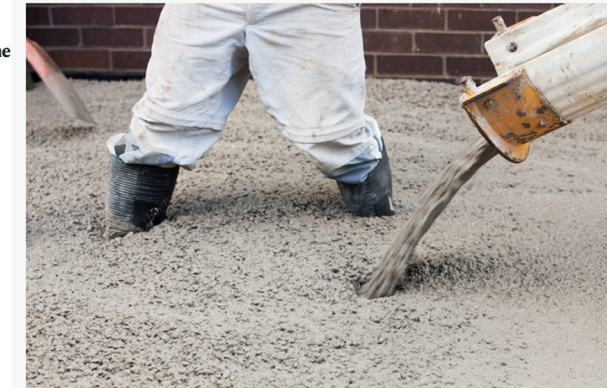
Pouring concrete for the floor of a house extension in Ambleside, UK. Credit: Ashley Cooper/Construction Photography/Avalon/Getty Images
